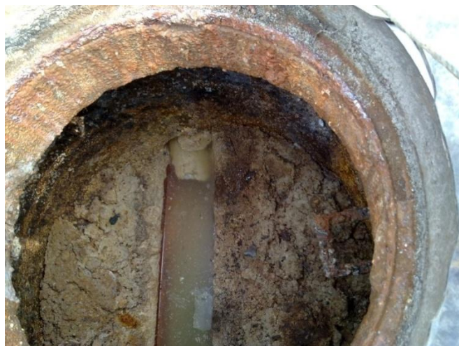
Fig. 1: FOG deposition at the Manhole.
